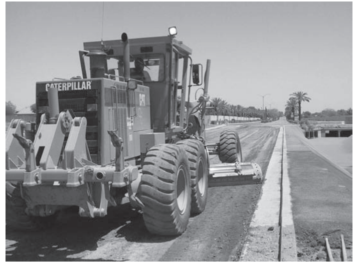
Critical infrastructure like roads, water lines, and fire stations are often built with bond financing.
