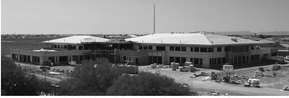
The Public Safety Administration Building going up immediately south of the city municipal complex will house the Police Department Headquarters & firing range, Fire Department Administrative offices, and a television studio for the city's Government Channel 11.
